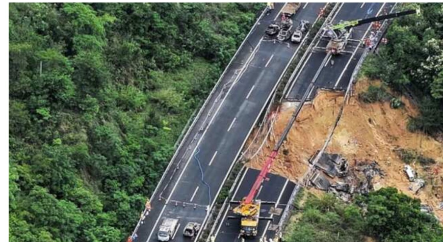
Rescuers work at a collapsed section of the Meizhou-Dabu Expressway in China's Guangdong province Photograph:(Others)
